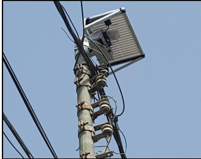
Figure 4. Data Logger installed at Clifton
